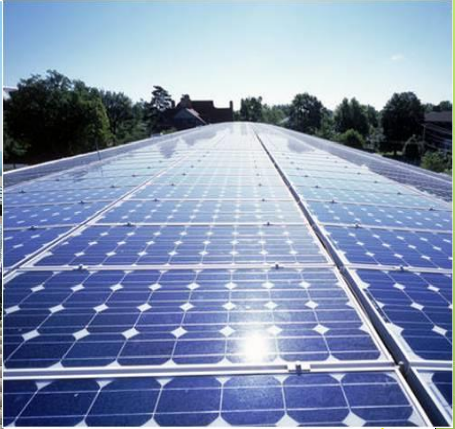
Solar Photovoltaic (PV)
